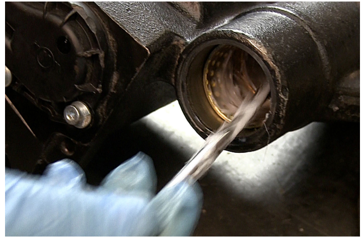
Figure 23. Using a brush, completely fill all dimples and grooves with Max-A-Sil 998™ grease.
